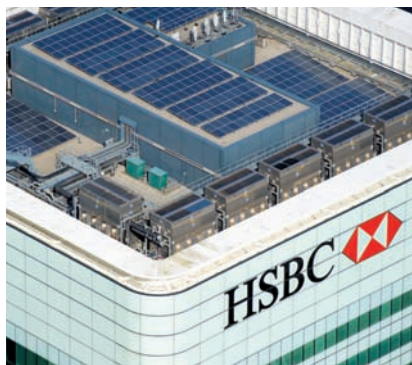
HSBC illustrates its commitment to supporting renewable technologies by installing solar panels at its Group Head Office in London.
